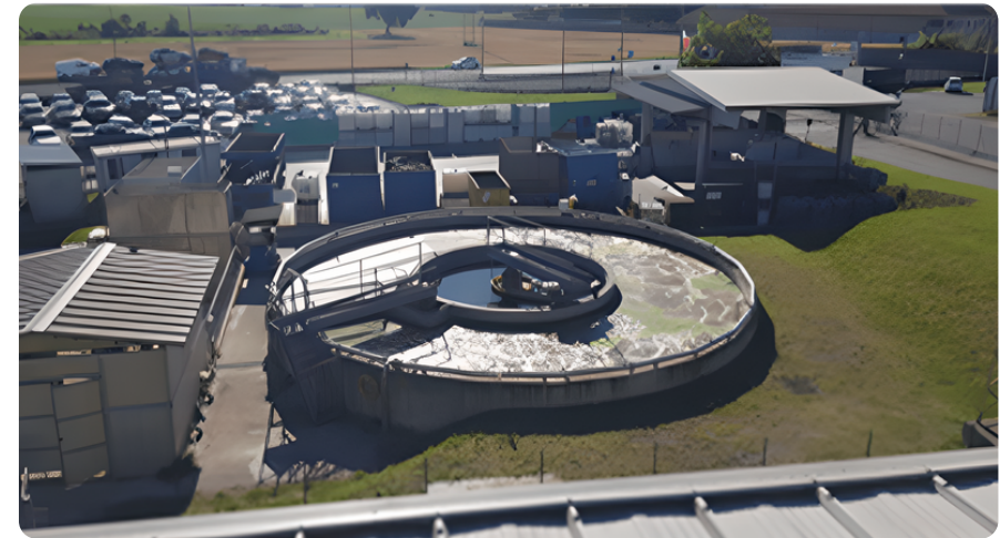
Water treatment equipment in CIR plant
